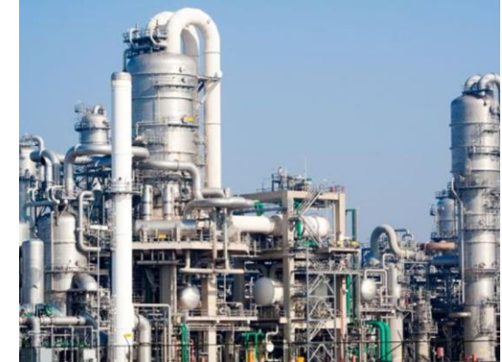
Process plant monitoring (DTS)
